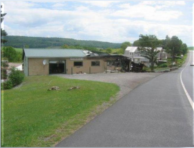
After the fire
