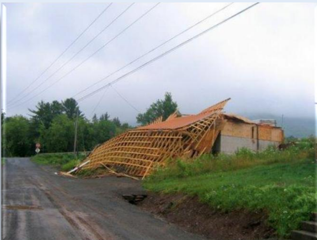
After collapse in a thunderstorm
